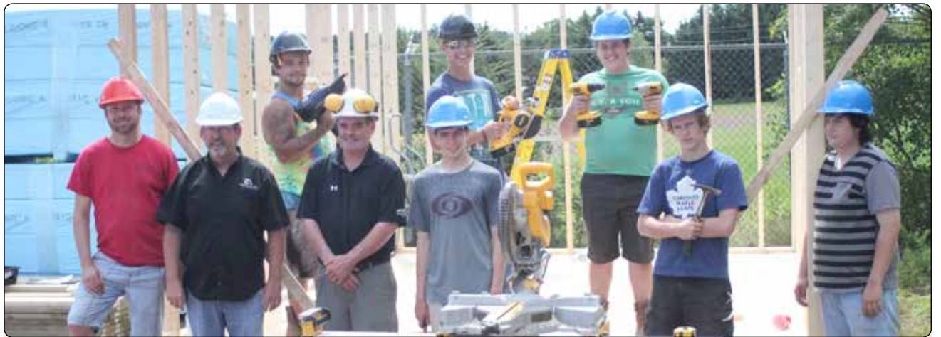
Participants of the Youth In Trades program in Charlottetown built a 12' x 16' storage shed on the premises of Castle Building Supplies. From left: Sandy Doucette, Program Facilitator, Sam Sanderson, Construction Association of PEI, Corey Doucette, Castle Building Supplies, and the program participants.
